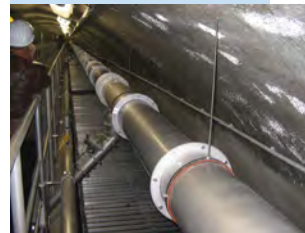
Concrete pipes with the lamella filter
