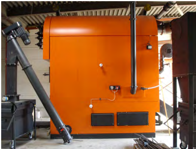
Wood chip-fired heating system at the BSR property on Gradestrasse
