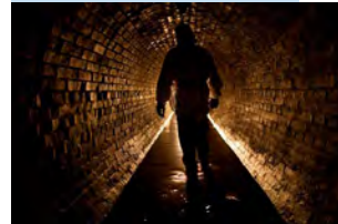
Accessible sewer system © BWB
